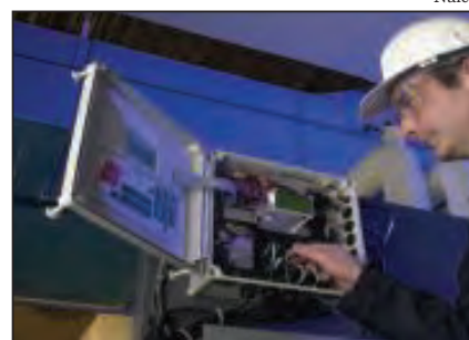
FIGURE 4. A technician looks inside a 3D Trasar Controller, which helps maintain control over critical cooling assets
