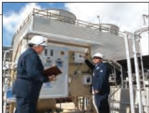
FIGURE 5. This image shows the 3D Trasar technology set up on a cooling tower.
