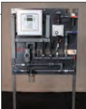
FIGURE 6. Here, the 3D Trasar technology is set up for a cooling water skid
